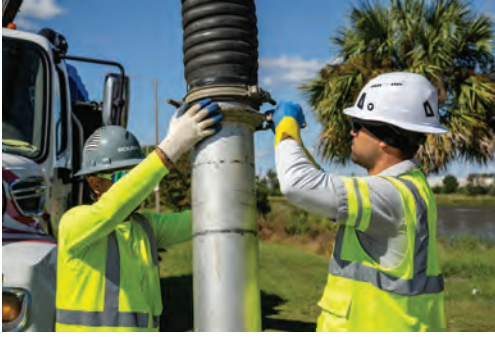
Gerson Arias (left) and Edear Urreabarre set up the vacuum boom to clean a storm line.
